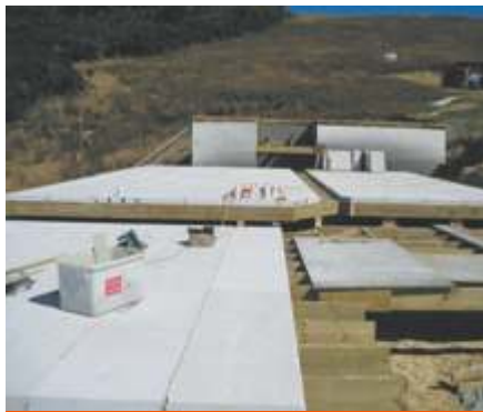
Fig. 10a : Hebel Power Floor at ground level.
